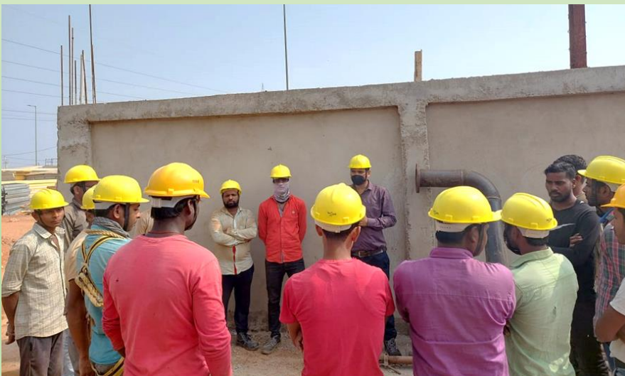
'Tool Box Talk' session is being conducted for all the workmen at TCW, Bhubaneswar (Project Site) on regular basis
